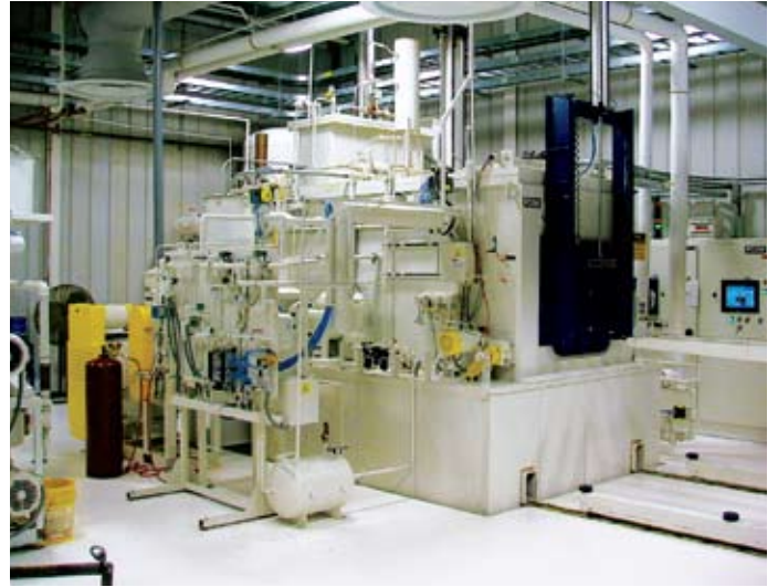
NHBB's vacuum carburizing furnace.
